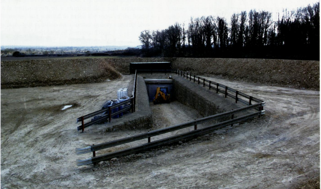
The new slope shaft into Park Lane Quarry, Corsham in late March 2013. Photo Dom Jackson
